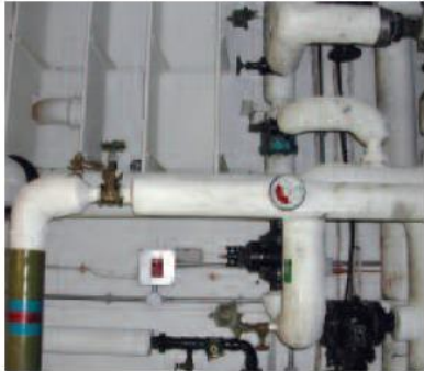
Asbestos insulation on pipes
