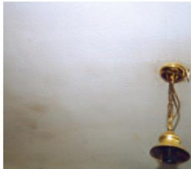
Textured coating with asbestos
